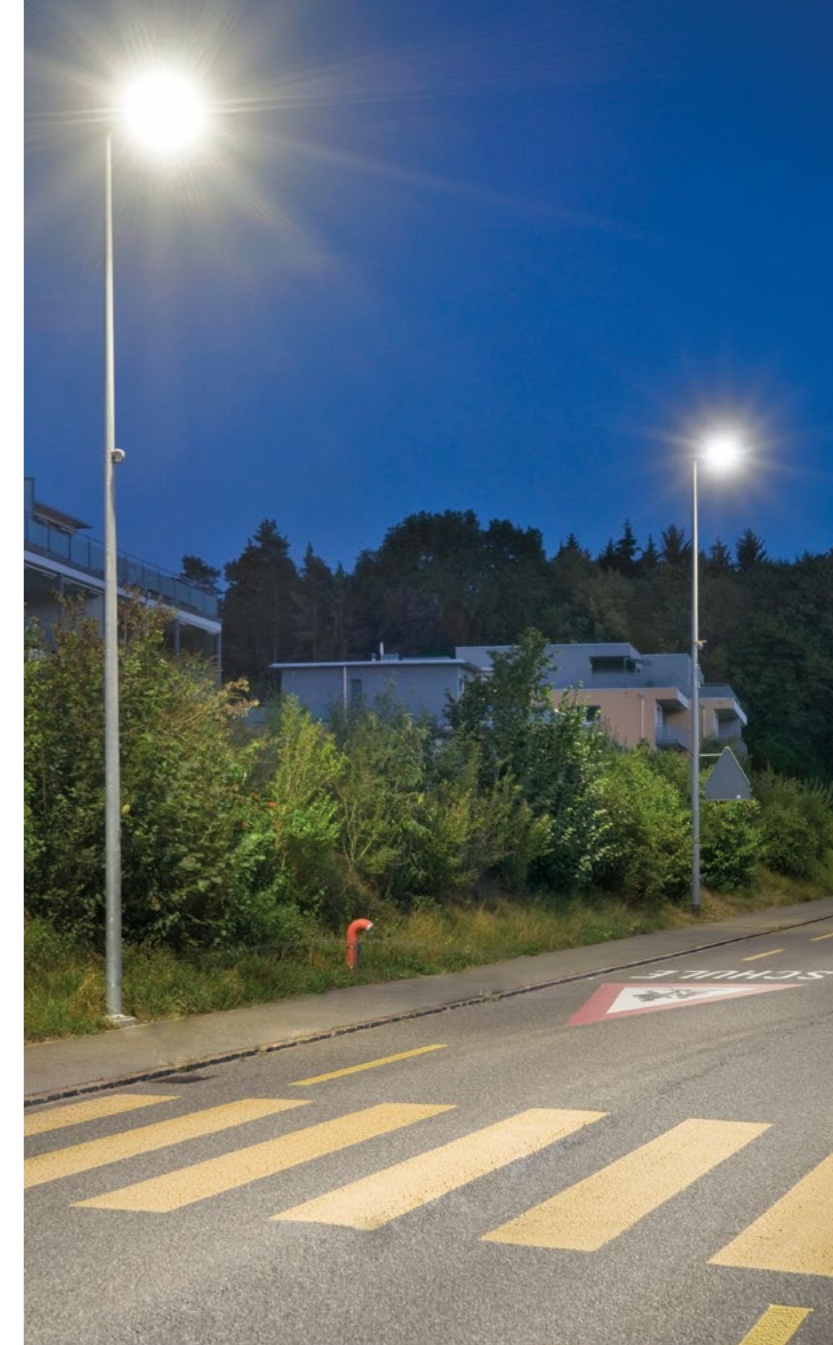
Streetlight 20 Aarau, Switzerland
